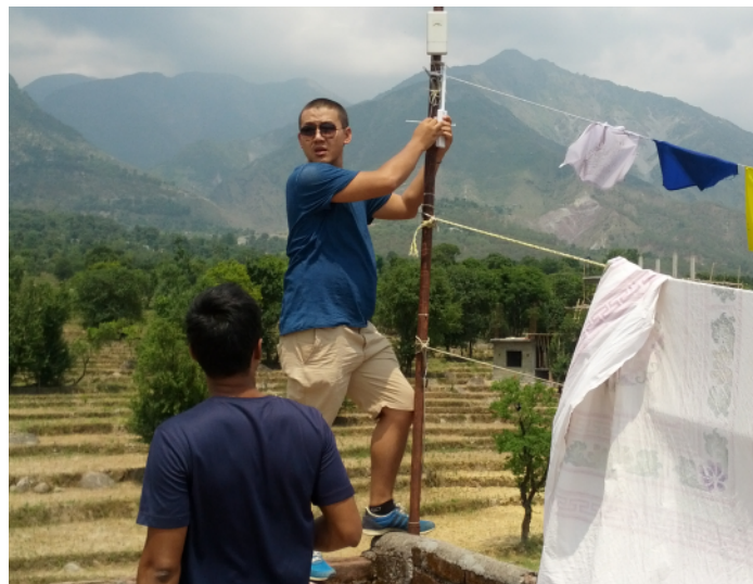
Connecting a PicoStation M2 unit to the mesh network.
